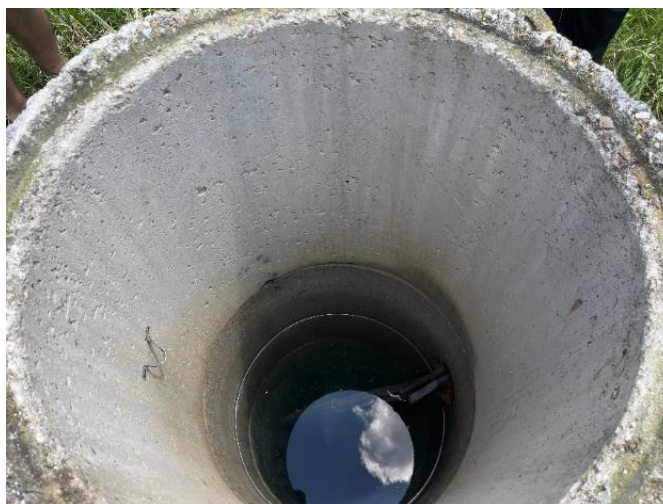
Figure 5. Water well in the village of Polac, Skënderaj
